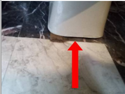
Recommend maintaining caulking at base of toilet.
