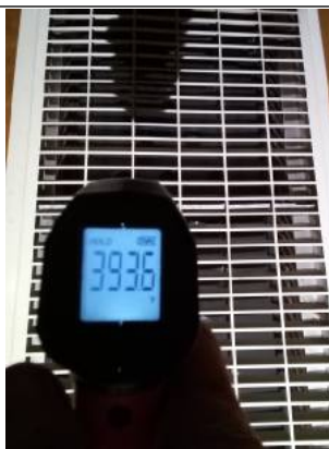
Temperature at wall heater.
