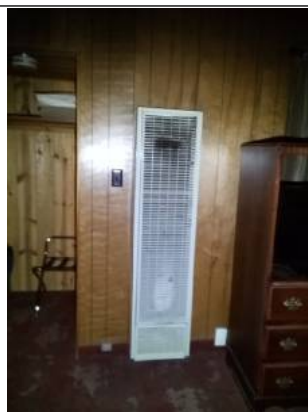
Call heater was tested and found to be in satisfactory condition at time of inspection.
