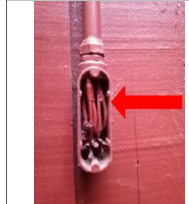
Mission cover recommend replacement to avoid moisture intrusion.
