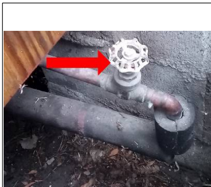
Shut off valve.
