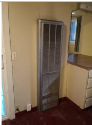
Wall furnace was tested and found to be in satisfactory condition at time of inspection.
