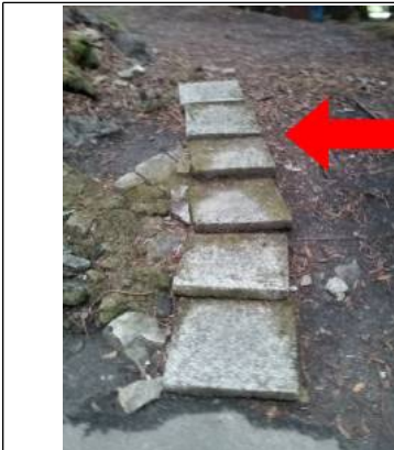
Uneven risers create a tripping hazard.
