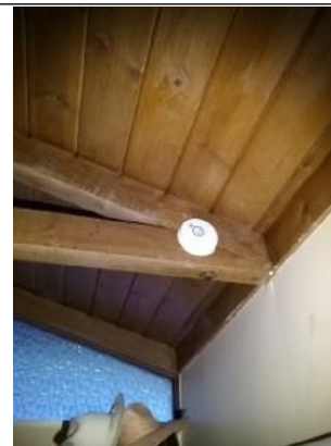
Smoke detectors were tested and found in satisfactory condition at time of inspection.
