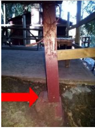
Settlement noted at post and Pier at corner of building recommend contacting licensed building contractor to evaluate and repair.
