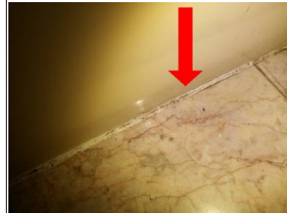
Recommend maintaining caulking at tub and floor junction to prevent moisture intrusion.
