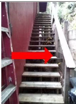
Recommend installing pickets and proper grab rails.
