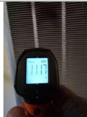
Temperature at wall heater.
