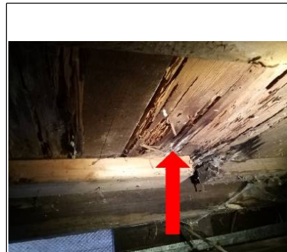
Moisture and pest damage.
