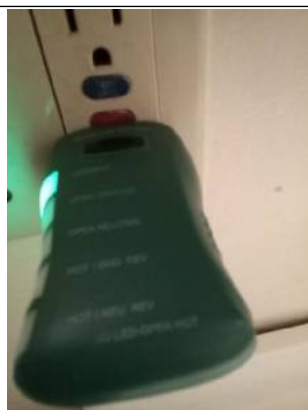
TFCI receptacle did not respond to testing. Recommend license electrician to evaluate and repair
