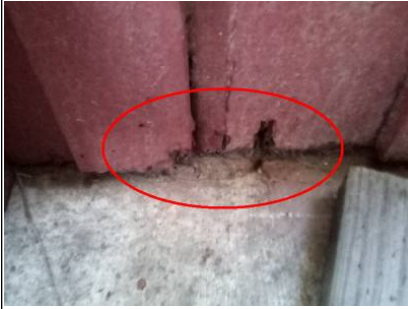
Dry rot and fungus damage.
