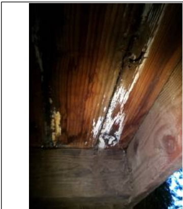
Fungus damage attack on cabin 9.
