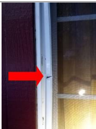
Bent and damage screen.
