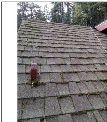
Moss build up
