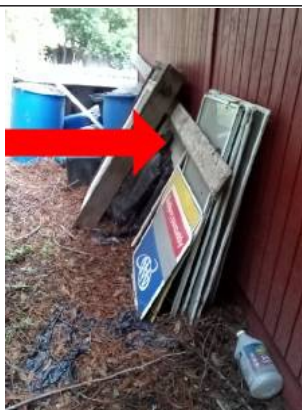
Recommend removing items from siding to prevent premature aging and deterioration.
