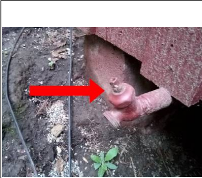
Hose bib missing handle.
