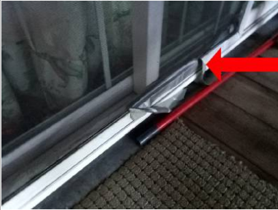
Damaged screen at patio door recommend repair.
