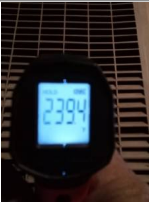
Temperature at wall furnace.
