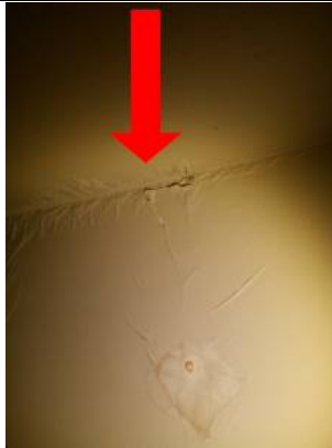
Damaged drywall ceiling recommend repair.
