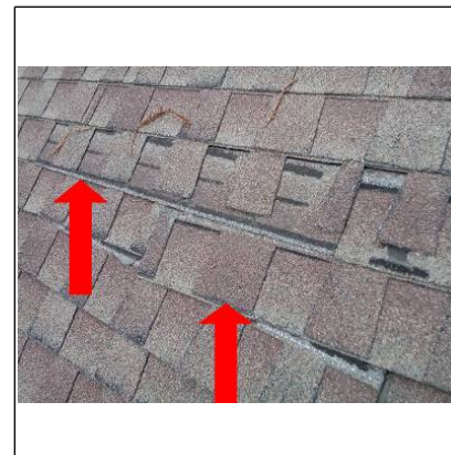
Loose mismatched shingles.
