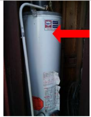
Recommend seismic strapping be installed.
