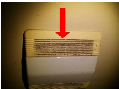
Recommend cleaning lint from exhaust grate.
