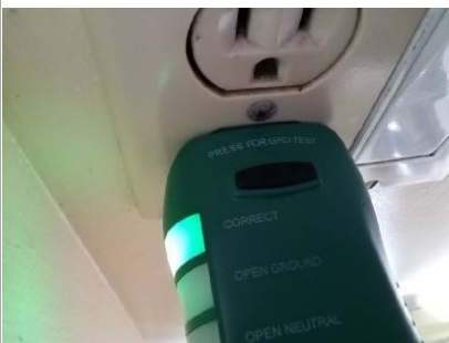
Recommend GFCI receptacles being installed in all bathrooms and kitchens this is a safety concern.
