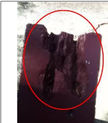
Dry rot fungus damage.
