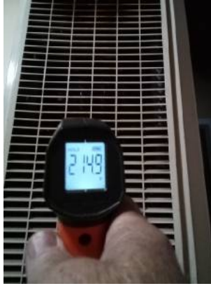
Temperature at wall furnace.
