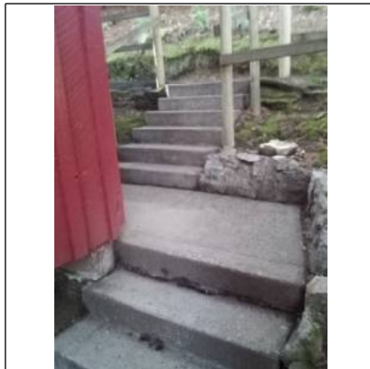
Steps at cabin 8
