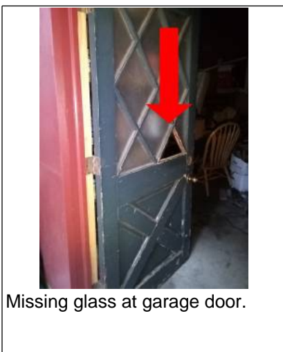
Fungus damage noted door jamb recommend repair or replacement.
