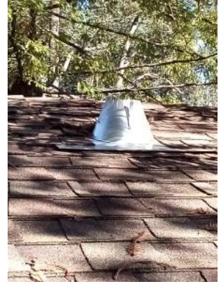
Missing cap at roof jack.
