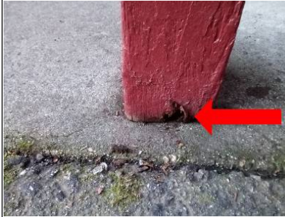
Fungus and dry rot damage on post at entry recommend contacting appropriate trays to evaluate and repair.
