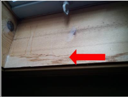
Moisture stains at skylight.
