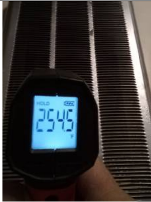
Temperature at wall heater.
