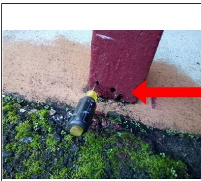
Fungus damage and dry rot at entry post recommend contacting appropriate trades for repair or replacement.
