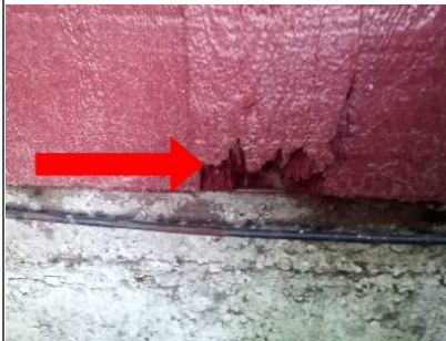
Try rot fungus damage at trim
