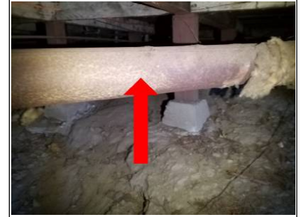
Insulation missing on ducting recommend replacement for better heat retention.
