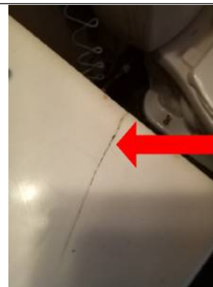
Crack and vanity top that bathroom.
