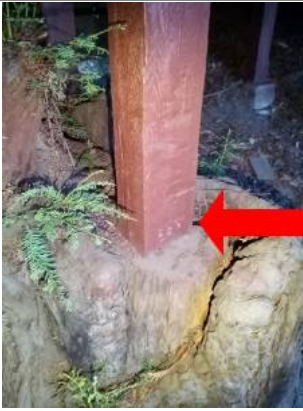
Improper support recommend contacting license building contractor to evaluate and repair.
