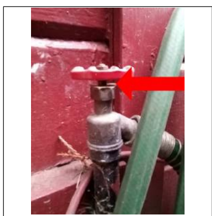
Hose bib leaking from stem.
