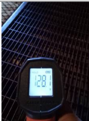
Temperature at floor furnace.
