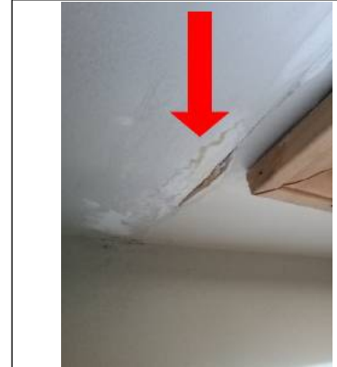
Drywall damage at ceiling recommend contacting appropriate trades for repair.
