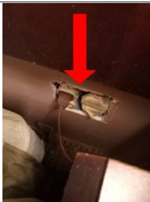
Missing outlet cover recommend replacement.
