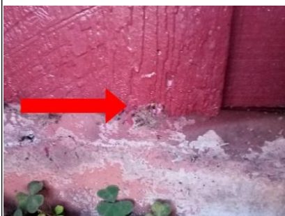
Dry rot damage it's trim.
