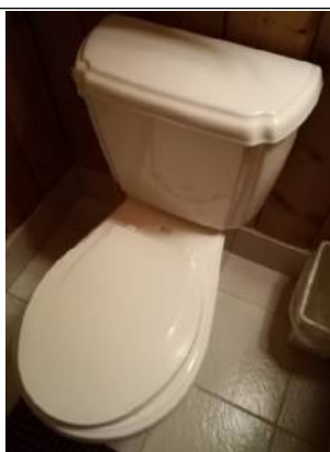
Low flow toilet noted.
