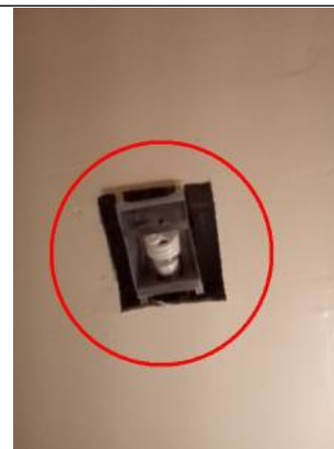
Missing grate at exhaust vent recommend replacement.
