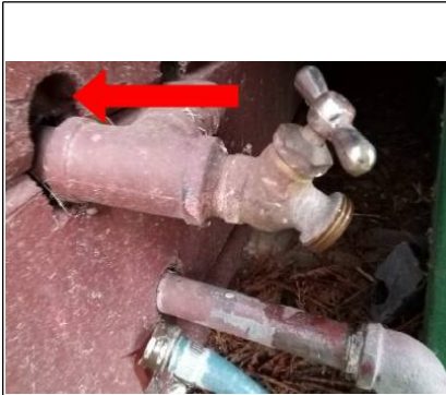
Recommend maintaining caulking at utility penetrations.
