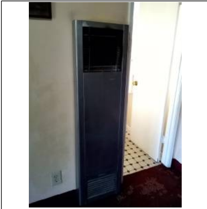
Well furnace was tested and found being satisfactory condition at time of inspection.
