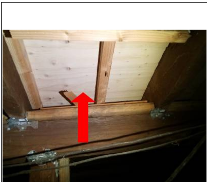
Subfloor repair noted.
