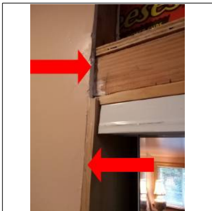
Trim and drywall missing at closet doors recommended repair and replacements.
